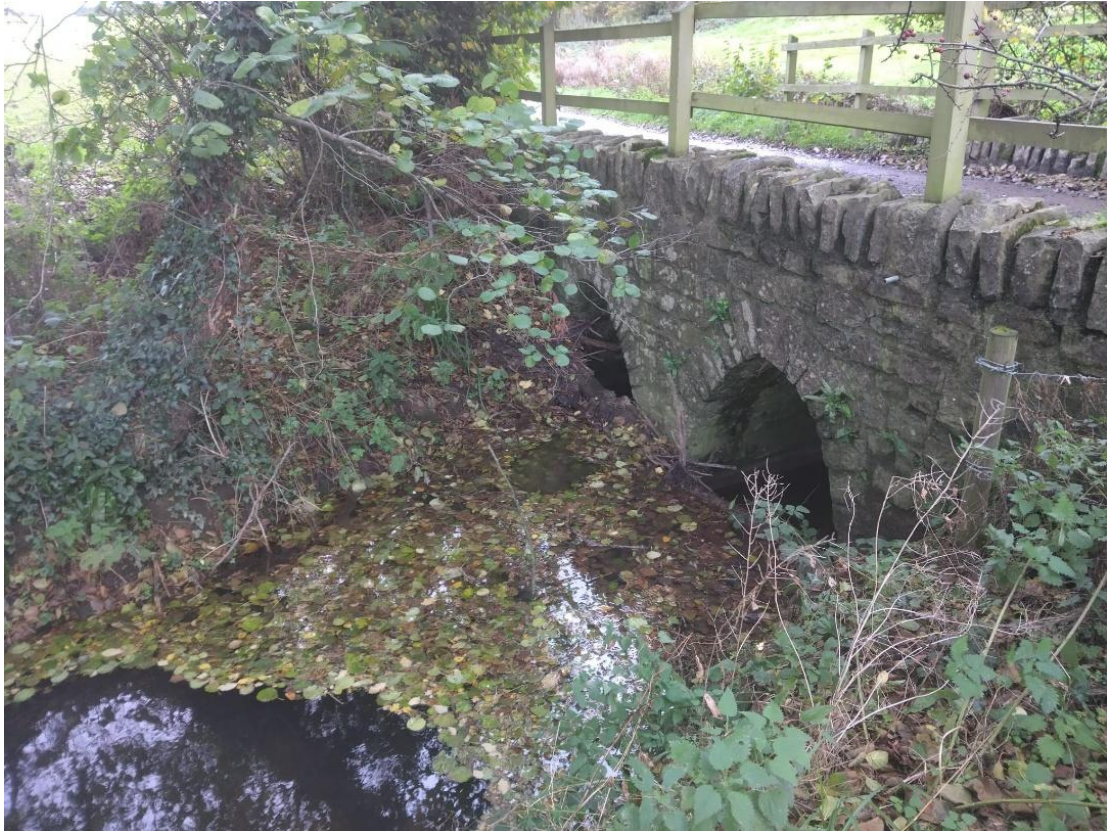
Debris accumulation at Sandbrook Lane Bridge
